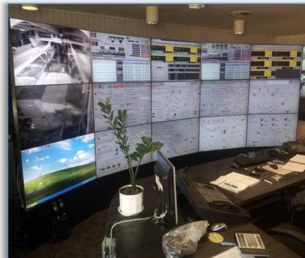
MCPD CONTROL ROOM
